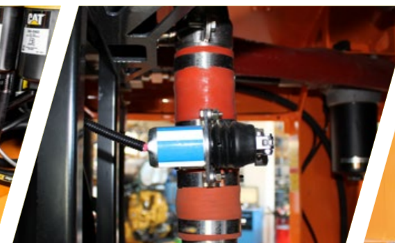
Air shut-off system
