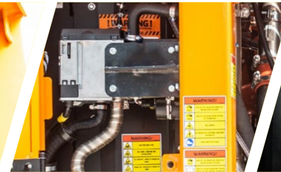
Pre-heating system for engine and hydraulic oil
