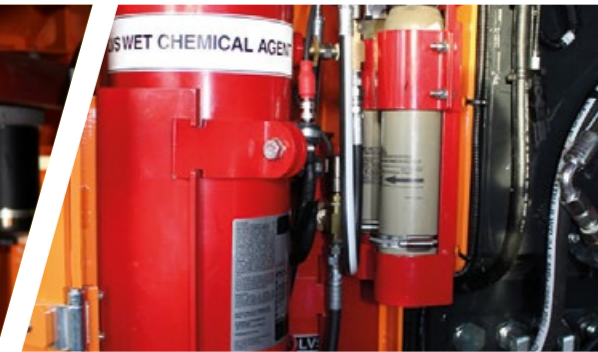
Automatic fire suppression system
