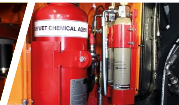
Automatic fire suppression system
